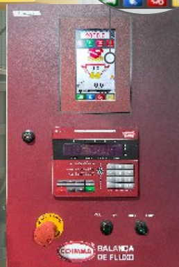
Painel de Controle
