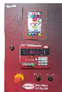
Panel de Control
